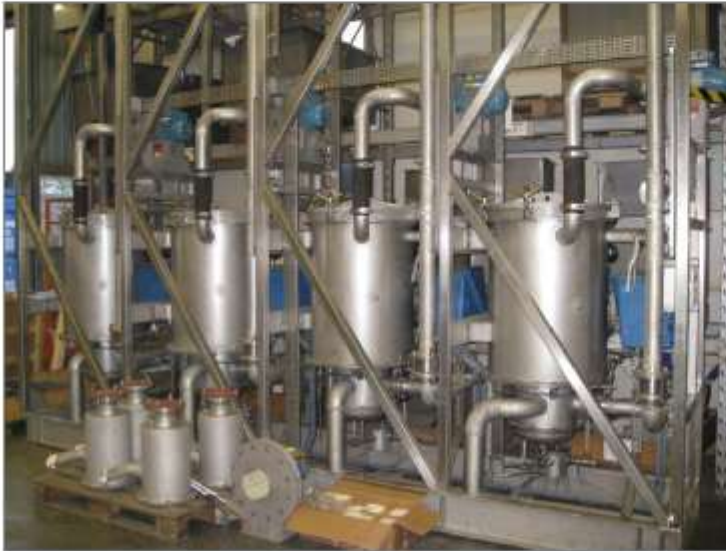
Four separators in one skid
